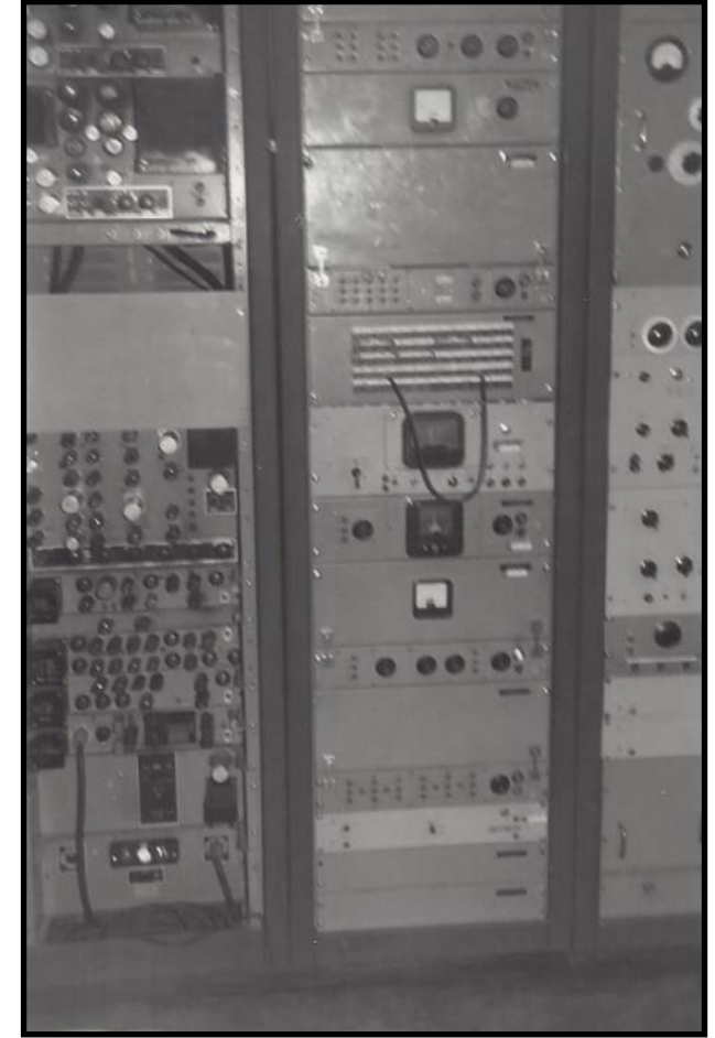
Sound patch bay and trap valve
