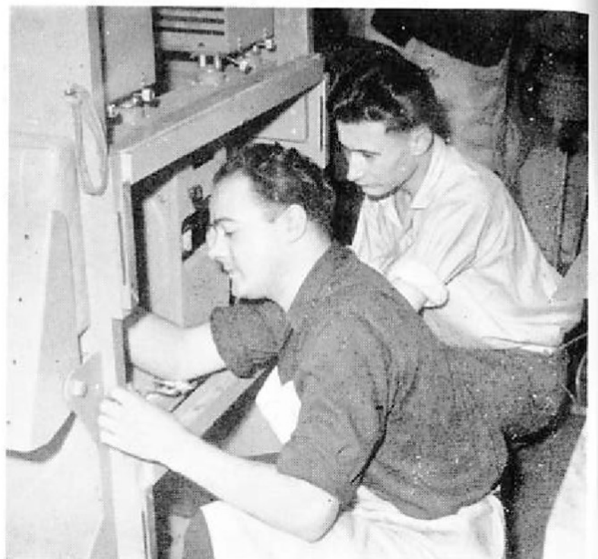
. . . Peter Barker and Dave Driver fixing cables to the "mousetrap" cable guides
