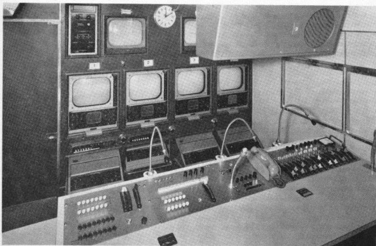
Fig. 6. A 12-channel Sound Mixer installed in an O.B van for Yugoslavia.
