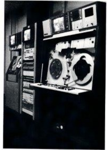
View of the B3410 Telecine and MR2B Video Tape Recorder installation recently supplied to Filmatic Laboratories, a leading specialist film-processing company.
