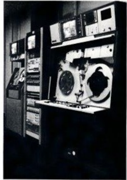
View of the B3410 Telecine and MR2B Video Tape Recorder installation recently supplied to Filmatic Laboratories, a leading specialist film-processing company.
