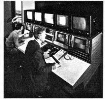
The switching centre undergoing final test at Chelmsford prior to its despatch to Abu Dhabi
