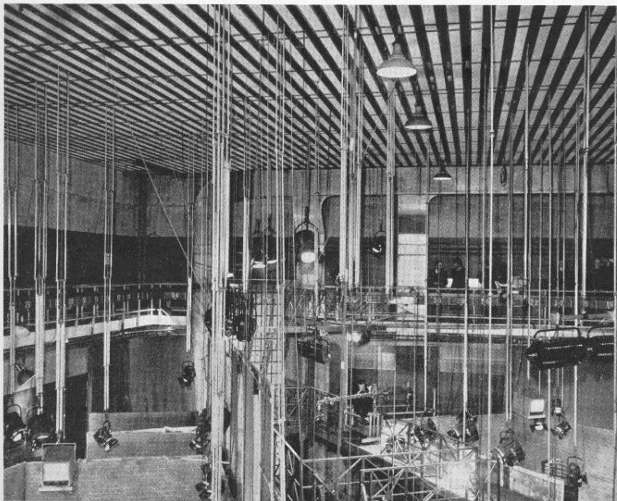
View showing grid structure and telescopic pendant assemblies supporting lanterns and monitors.
