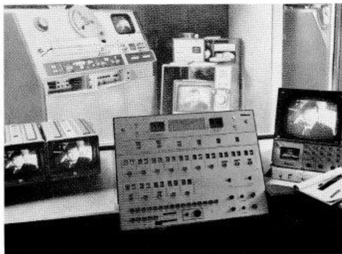
Assignment control in the VTR area. Panel provides source and destination monitoring and assignment indication.
