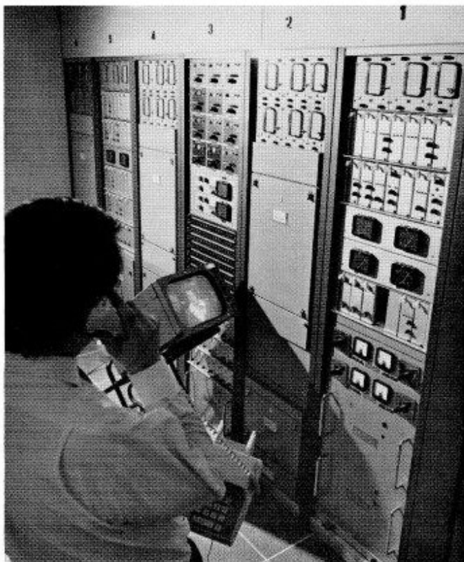
A clean air conditioned environment is required for maximum stability and reliability of equipment.
