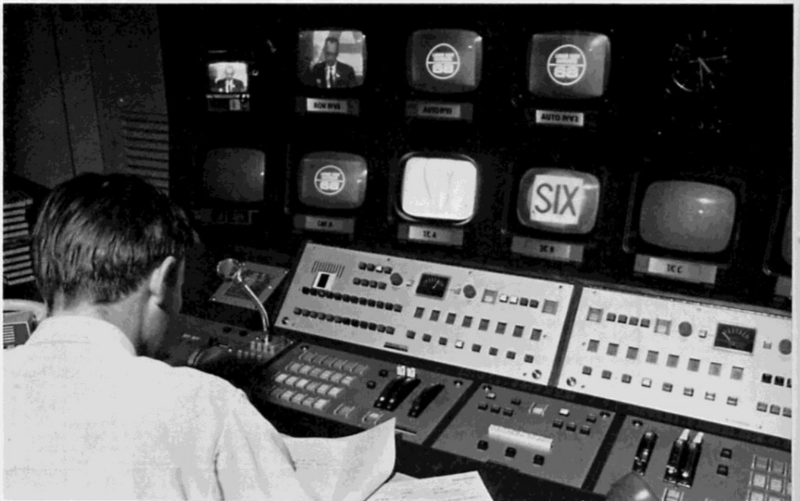
Fig.2 A general view of the Central Control Room.
