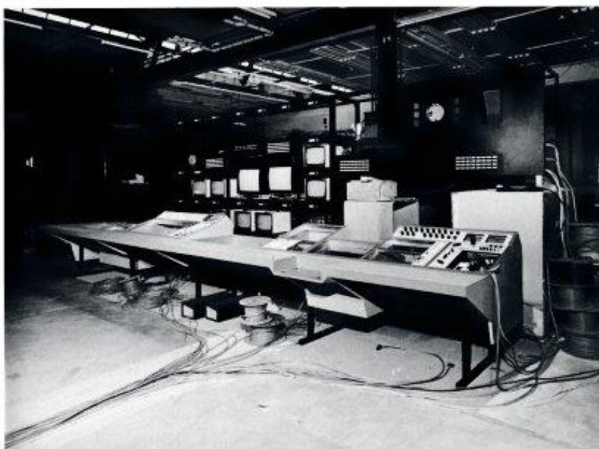
Fig. 2. The control desk and monitor stack assembly for the production control room being pre-assembled at Marconi's Chelmsford factory
