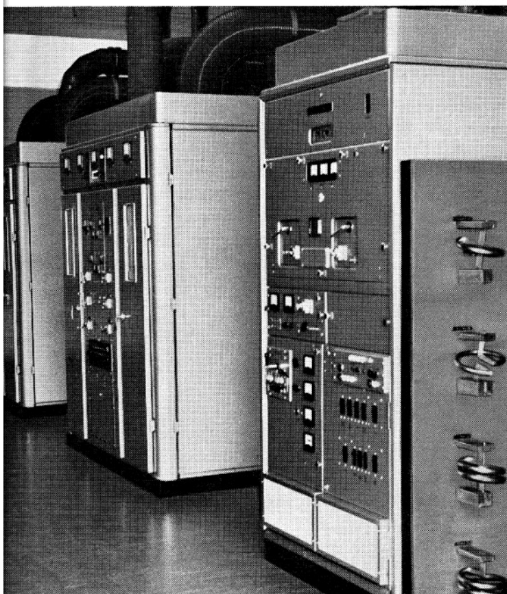
Fig. 7. One of the two 250-kW transmitters.
