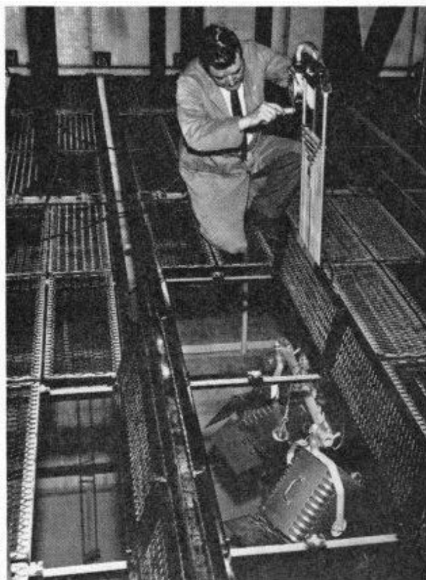
Fig. 8. The upside down grid at Television Wales and West. Though this system requires longer hangers from the roof beam, it is a very convenient method. The loading gallery can be seen through the trap doors in the planks.
