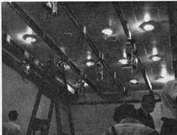
Fig. 10. A bus-bar suspension system at Shell Centre, London. In this system, power is fed through the suspension bars and the lights are hung on lazy tongs.
