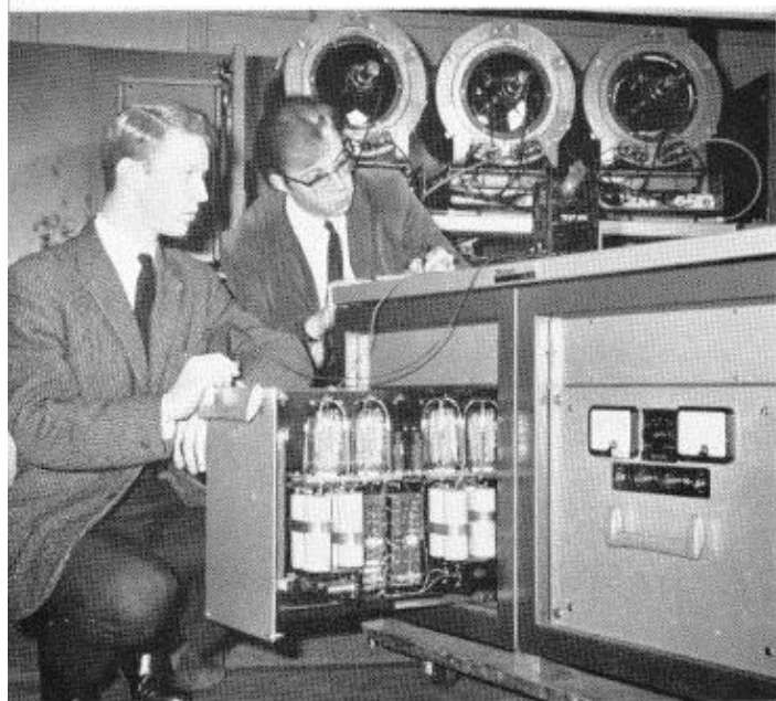
Apprentices Malcolm Davies and Paul Webber checking the power supply cabinet for the large screen colour projector
