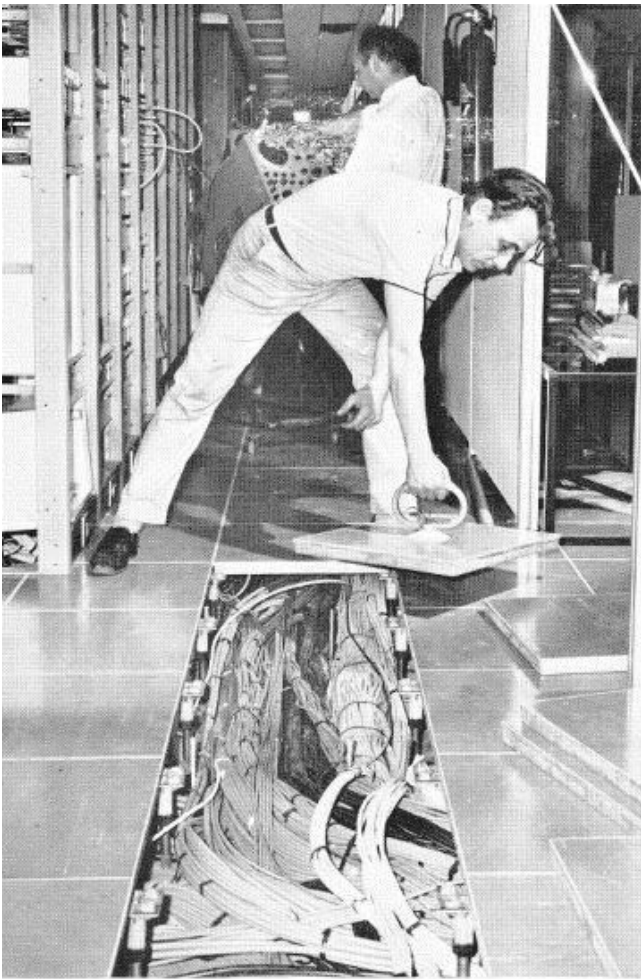
One of the contract wiremen lifts computer floor tiles to reveal some of the cables which carry video, audio, and other electrical sources throughout the station. He uses a special suction lifting pad for speed
