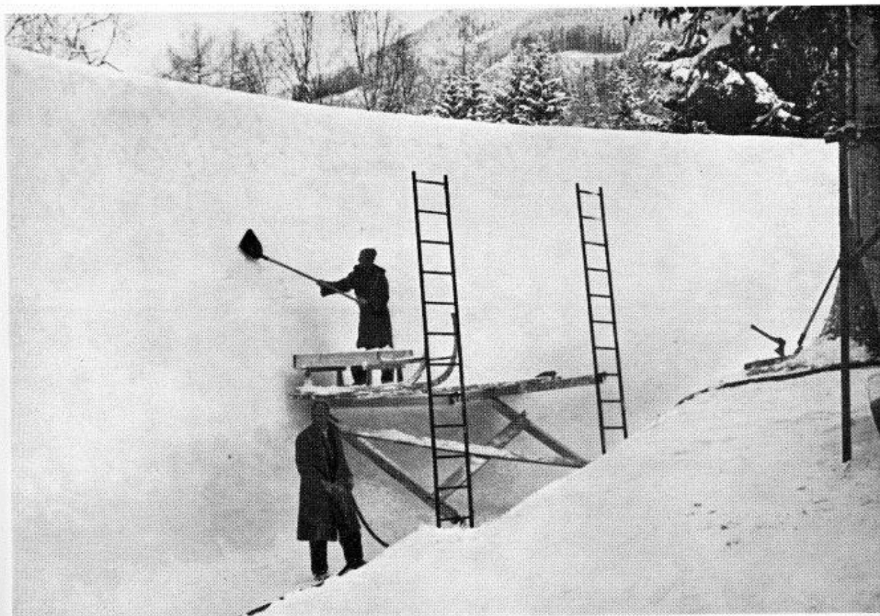
Fig. 5. Building up the bob-way walls. Camera scaffolding can be seen at the right.
